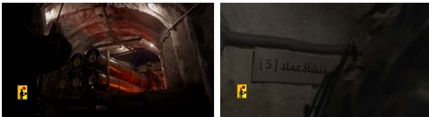
Right: A sign reading "Imad 5 Facility" (Hezbollah combat information Telegram channel, November 3, 2024). Left: Six missiles moments before being elevated to ground level via a track system. (Hezbollah combat information Telegram channel, November 3, 2024)
