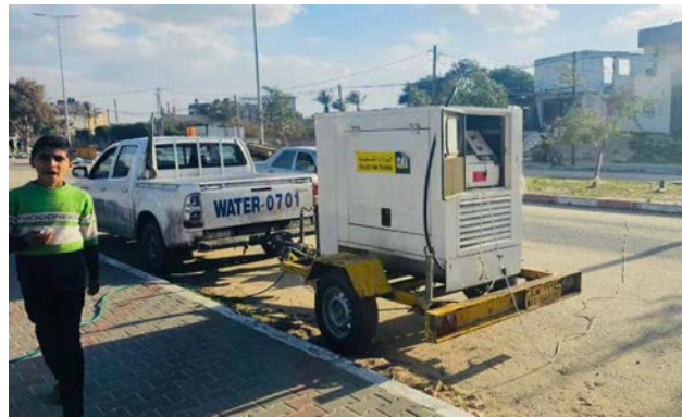
The municipality operates wells for the benefit of the residents (Khan Yunis Municipality Facebook page, February 3, 2024)
