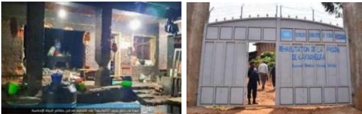
Right: The entrance gate to the prison (the UN website, December 13, 2016). Left: The prison after the break-in of ISIS operatives (Amaq, August 12, 2022)
