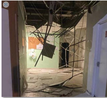
Some of the damage caused by the explosion in the hospital in Nabatieh (Lubnan24, February 7, 2023)
