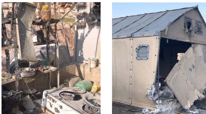
Makeshift structures damaged by the attack on the displaced person's camp (Hadi@HadiAlabdallah Twitter account, November 6, 2022)
