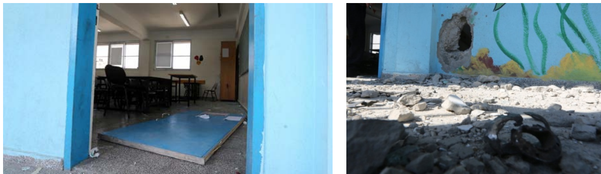
Damage done to the UNRWA school (Palinfo, August 13, 2020).
