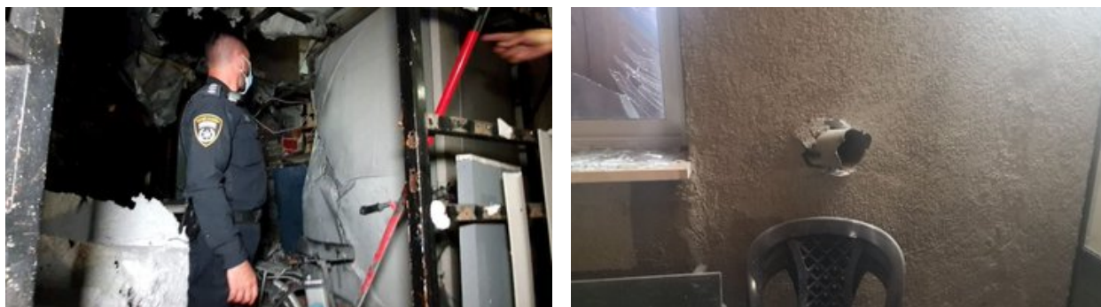
The house in Sderot damaged by a rocket (Twitter account of journalist Hassan Aslih, August 16, 2020).
