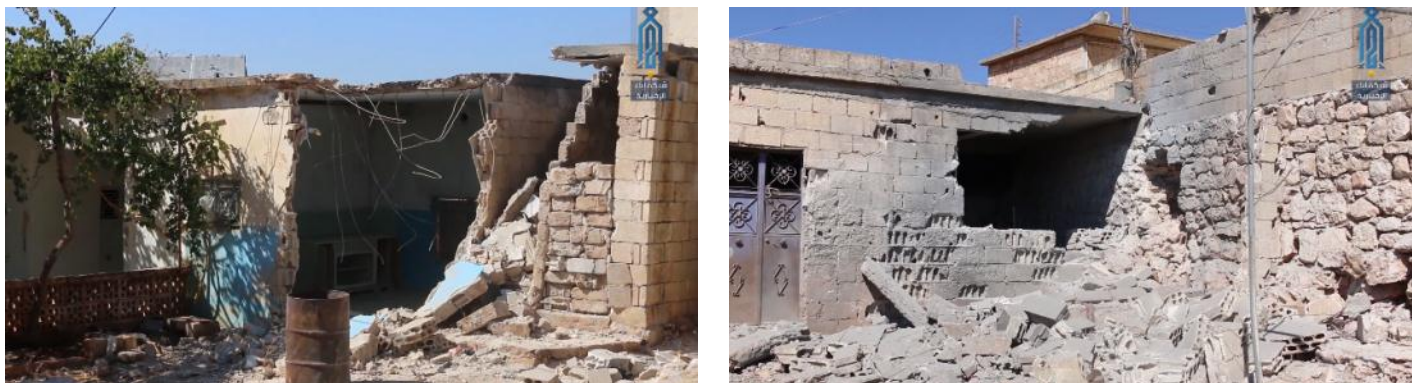
Buildings at Kafr Oweid southwest of Idlib, hit by Syrian army artillery (Ibaa, September 28, 2019)
