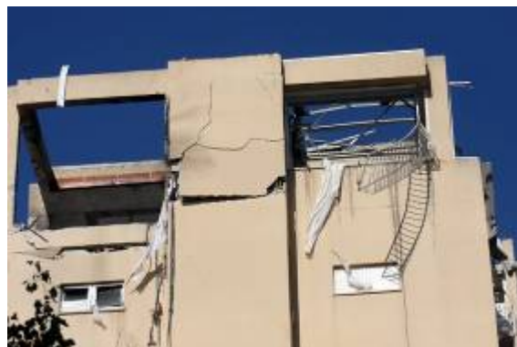
Apartment house in Ashdod takes a direct hit on January 1 (Roei Idan for the Sderot Media Center, January 1, 2009).
