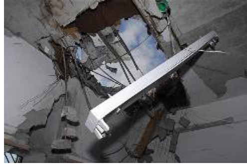
The hole ripped in the roof of a school classroom (Photo by Herzl Yosef, Ynet, December 30).
