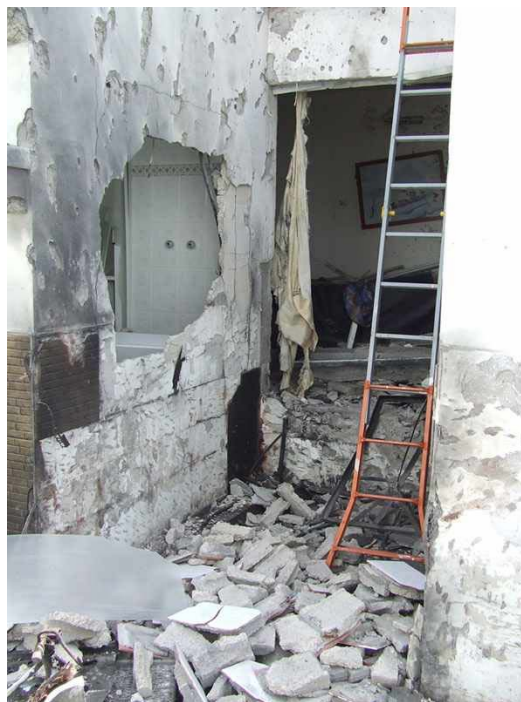
A house in Sderot destroyed by a direct rocket hit (Photo courtesy of Sderot security staff, May 16)
