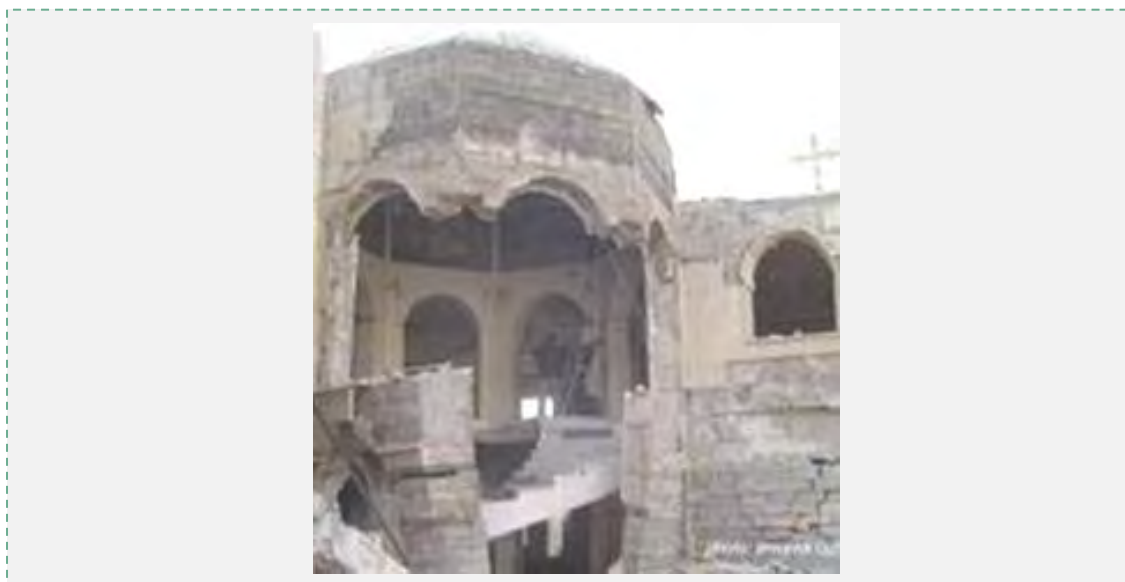
A Mosul church vandalized after ISIS occupation the city in June 2014. The media claimed that it had been demolished by IEDs (Abnar.ir).
