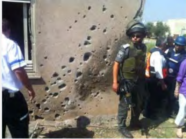
Damage to a residential structure in an Israeli town (Daniel Hajbi for the Sderot Media Center, June 20, 2012).
