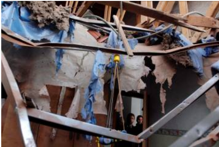
A house in Sderot damaged by a Qassam rockets (Amir Cohen for Reuters, January 15).
