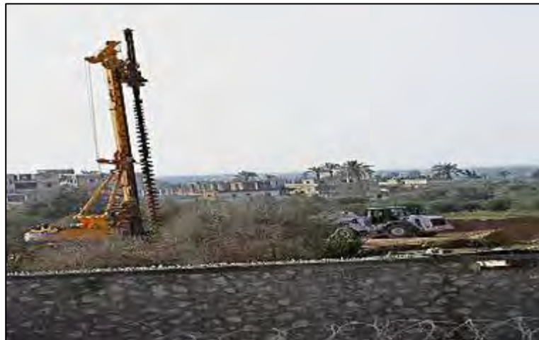
Egyptian excavation works in Rafah for the construction of the barrier (Felesteen, December 18, 2009)
