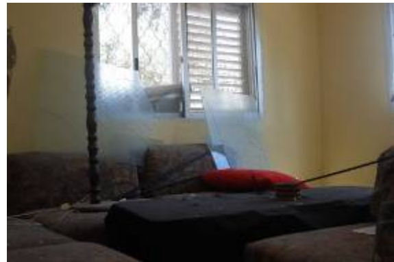
A house in Sderot damaged by rocket fire (photo by Hamutal Ben-Shitrit, www.sderotmedia.com , June 24)
